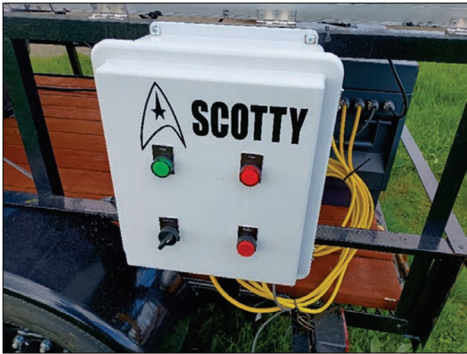
Close-up view of the SPOC control panel (Photo credit: Doug Berwick, Jacobs)
