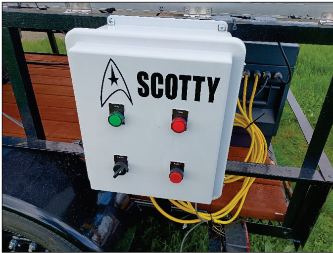
Close-up view of the SPOC control panel (Photo credit: Doug Berwick, Jacobs)
