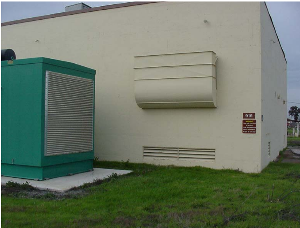
Photograph 2: Southeast Corner of Installed Generator at SD043.
