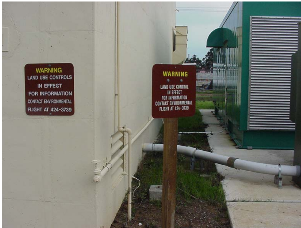
Photograph 3: Generator Pad and Warning Signs at SD043. Stanchion of Former Pad with Leaking Transformers is visible in the foreground.
