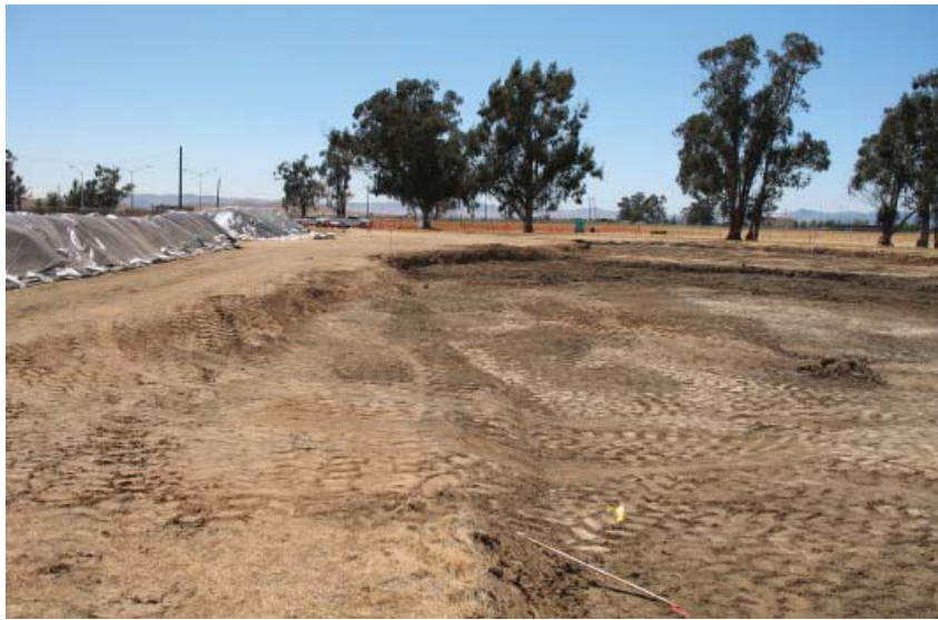
A large excavation void remains after the cleanup of a former small arms range is complete. Note the covered stockpiles of contaminated soil that will be sent to a designated soil repository.
