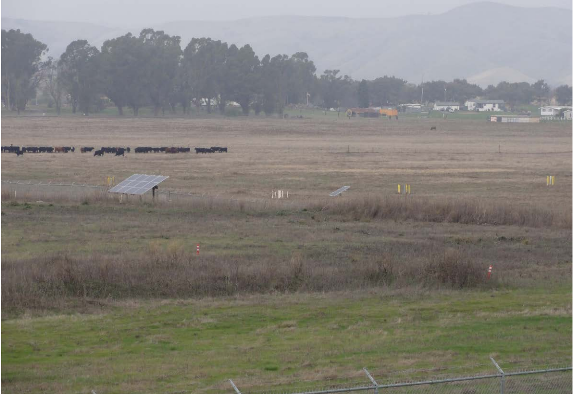
Photograph 8: LF007 Solar Panels [NW]
