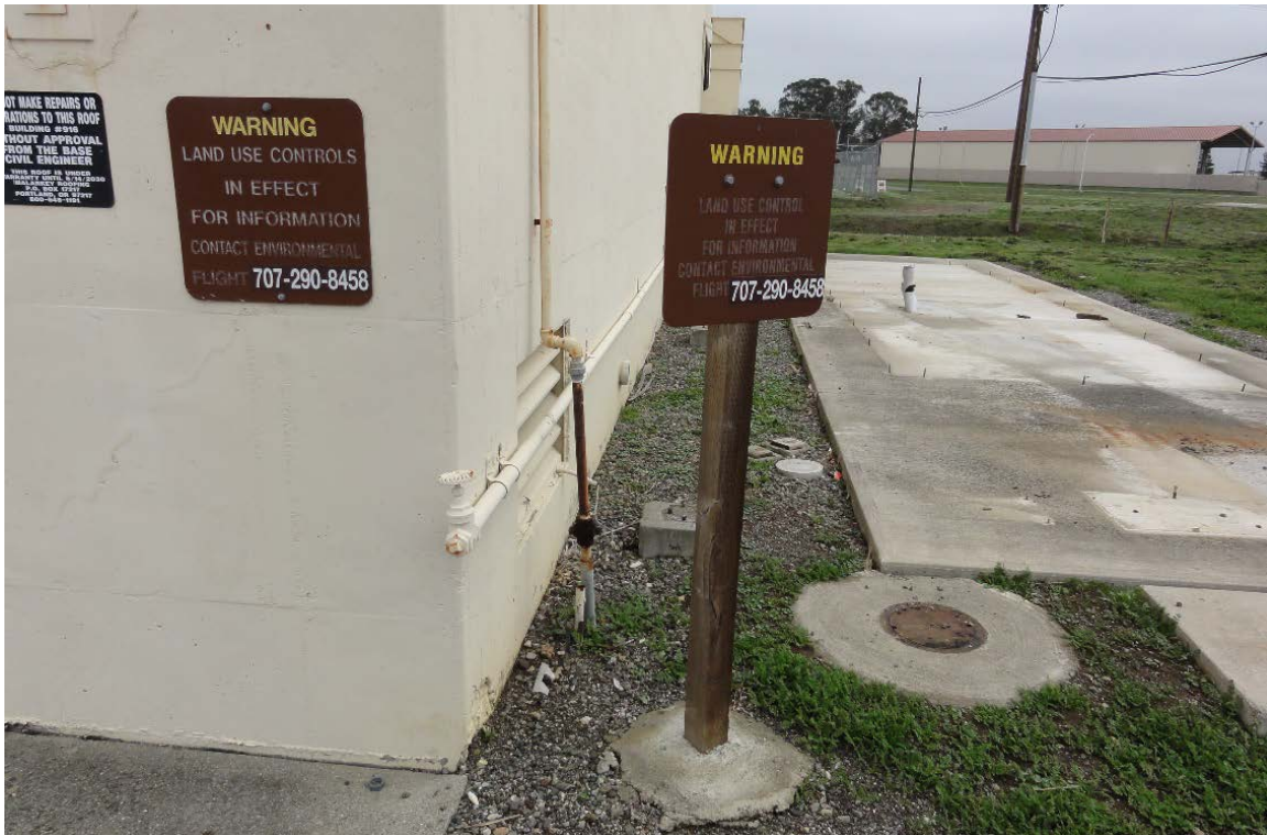
Photograph 32: Generator Pad and Warning Signs at SD043. Stanchion of Former Pad with Leaking Transformers is visible behind the warning sign post. Generator has been relocated. [E]
