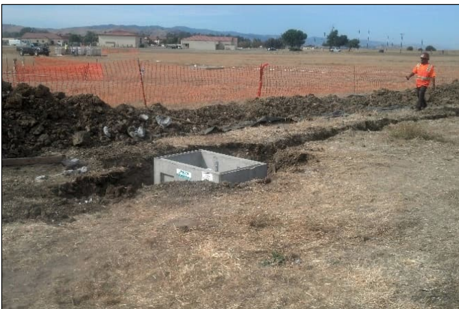
Figure 6. Photo of the installation of the concrete vault for an extraction well. (Photo credit: Jacobs)
