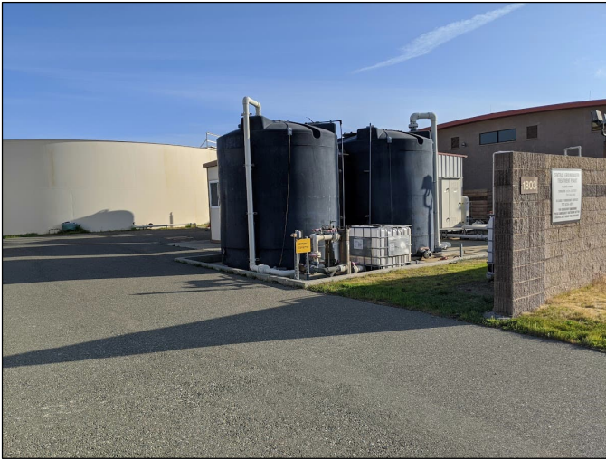
Entrance to the Central Groundwater Treatment Plant. Two groundwater holding tanks are shown, with the large treated water holding tank (back left) and neighboring fire station (back right) shown as well. (Photo credit: Doug Berwick, Jacobs)
