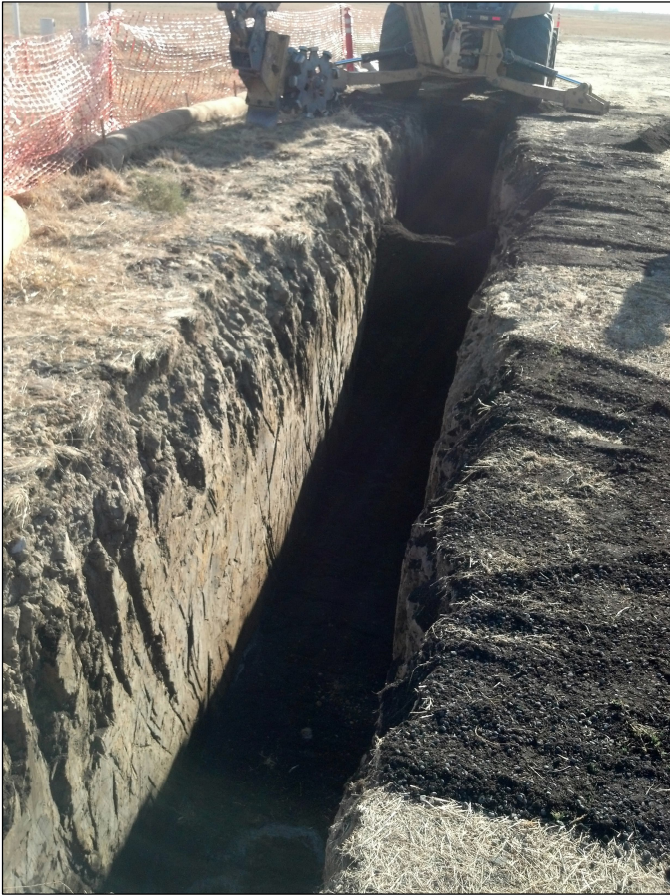
Figure 5. Photo of the bioreactor trench backfilled with the gravel, mulch, and pyrite sand mixture. (Photo credit: Jacobs)
